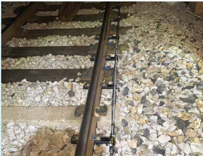
Monitoring for railways | Ballasted track
