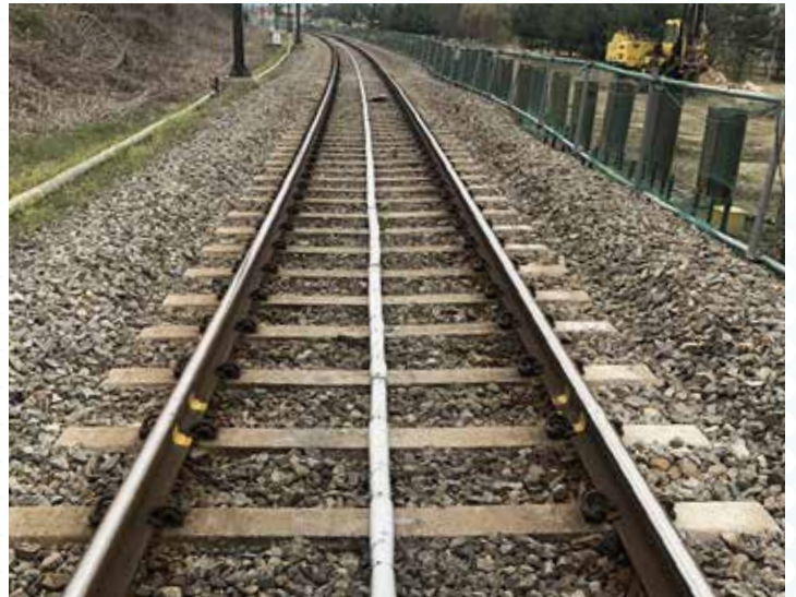
Monitoring for railways | Ballasted track
